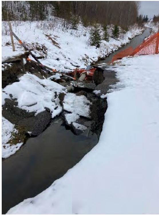
Photograph 3: Damages caused by flooding at Site 2
