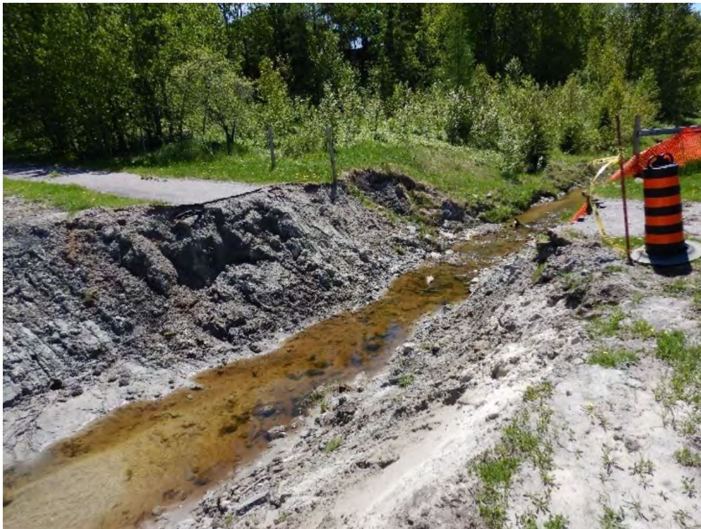
Photograph 4: Site 2 after cleanup. Culverts and asphalt to be installed in order to restore site to original state.
