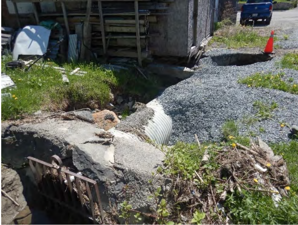
Photograph 5: Damage caused to culvert by flooding at site 3.
