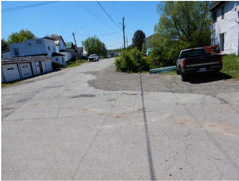
Photograph 7: Recycled asphalt placement after rip-rap removal and backfilling with granular 'A'. Same location of Photo 6.
